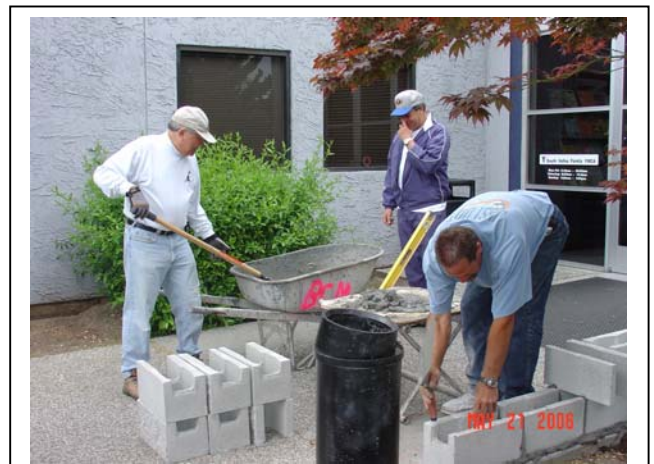
Bob Bloomfield , pictured here, laying the cinder blocks for the planter area. Bob , of Bloomfield Custom Masonry, donated his time and expertise to the project.
